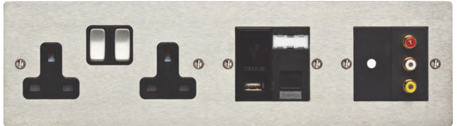
Double Switched Power Socket, RJ45, Telecom and AV/Data Sockets
