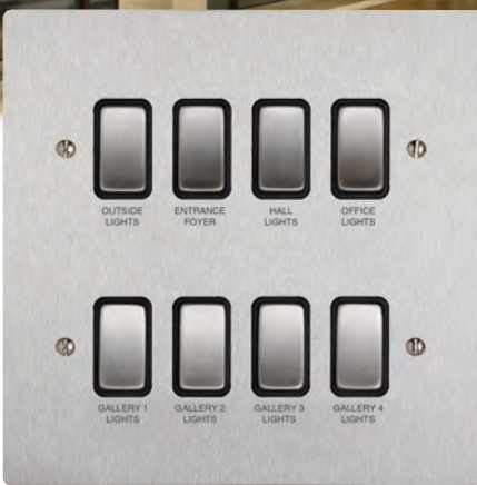
Gallery Utility Switches
